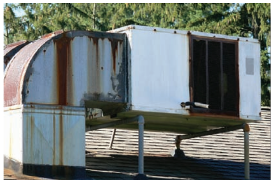
Roof top air handler
